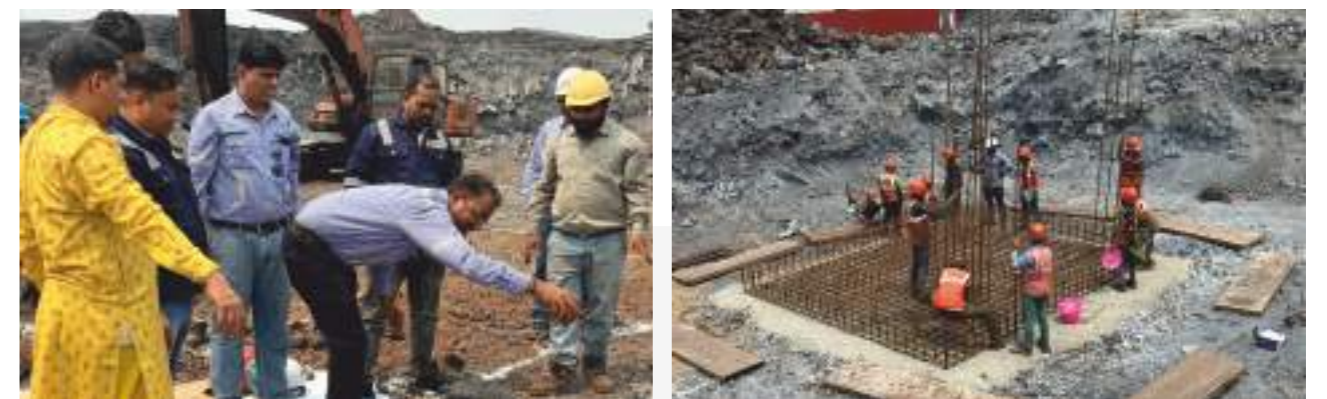
Puja and jubilant start of the construction phase of our Metal Recovery plant at Jharsuguda branch (K-JBPSL)
